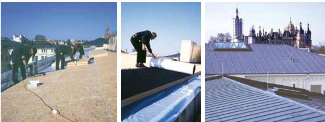
LINITHERM PAL OSB under the titanium-zinc roof of the historic stables in Schwerin
